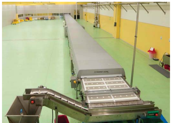
Antonio Agostoni checks on the production of chocolate chips on the newest moulding line installed in the facility, which features a 1.5-meter depositor and a cooling tunnel.
